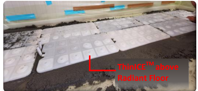
PCM (Hydrated Salt) installed above the radiant floor
