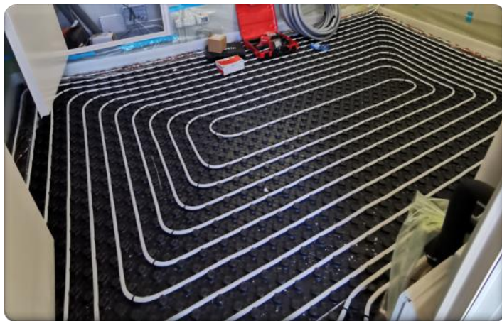
Radiant Floor Loop
